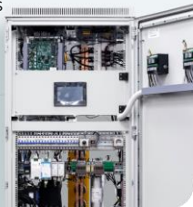
UNINTERRUPTIBLE POWER SUPPLY UNITS
