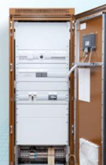
CHARGING AND RECTIFYING DEVICES
