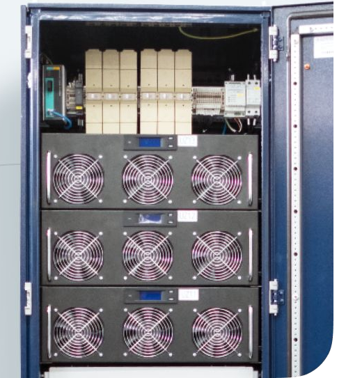
MODULAR UPS UNITS
