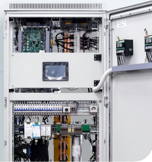
UNINTERRUPTIBLE POWER SUPPLY UNITS
